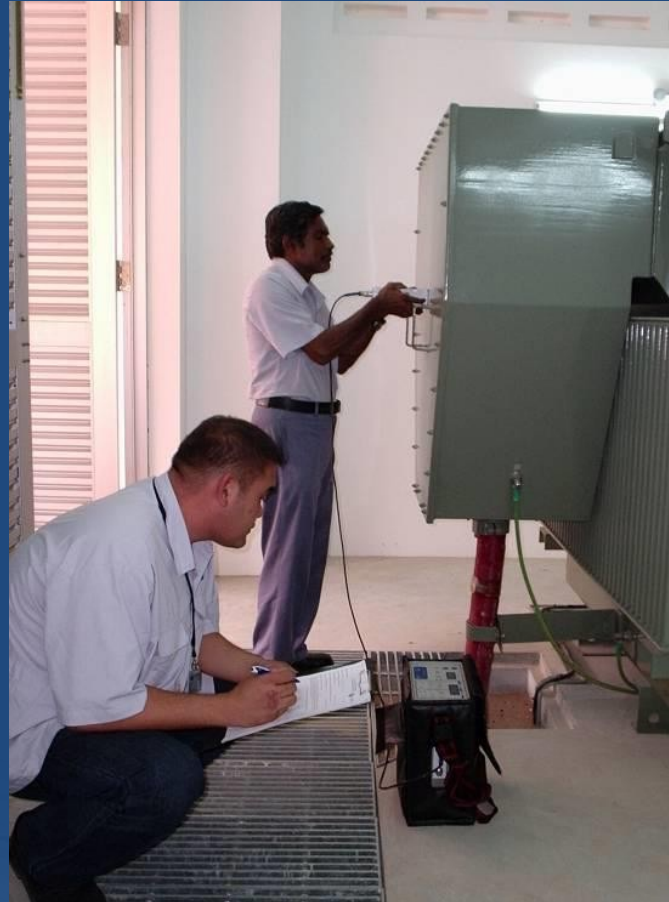
TEV Partial Discharge detection
