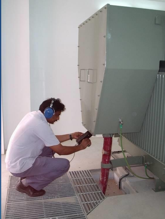
Acoustic Partial Discharge detection
