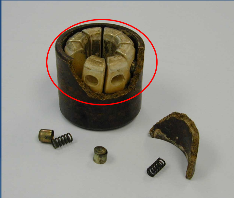
Faulty tulip contact assembly
