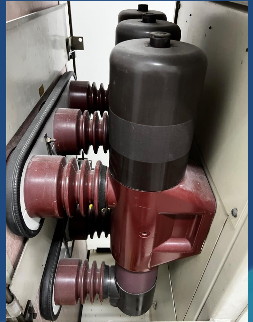
Oil-filled Circuit Breaker
