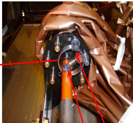
Broken Metallic Ring at Tap Changer
