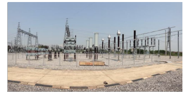
230 kV C-Bank, EGAT For utility grids
