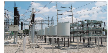
115 kV C-Bank, EGAT For utility grids
