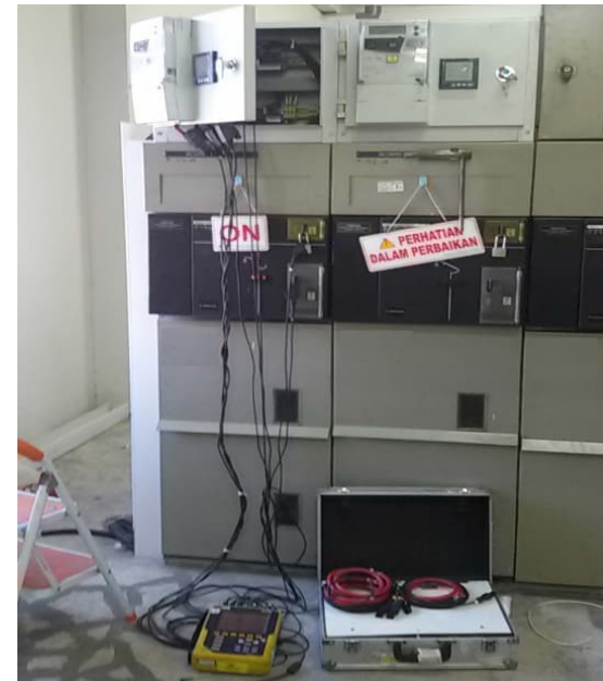
Measurement at 20kV
