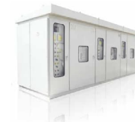
22/33 kV C-Bank, PEA
